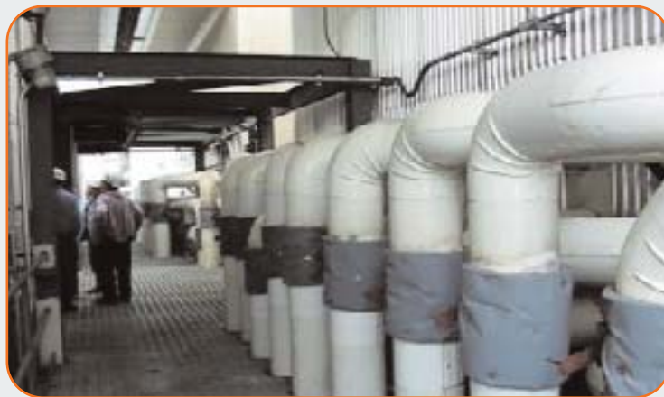
At Dynege's Baldwin Energy Complex, optimization has helped reduce SCR-related ammonia usage by 15 - 20 percent.
