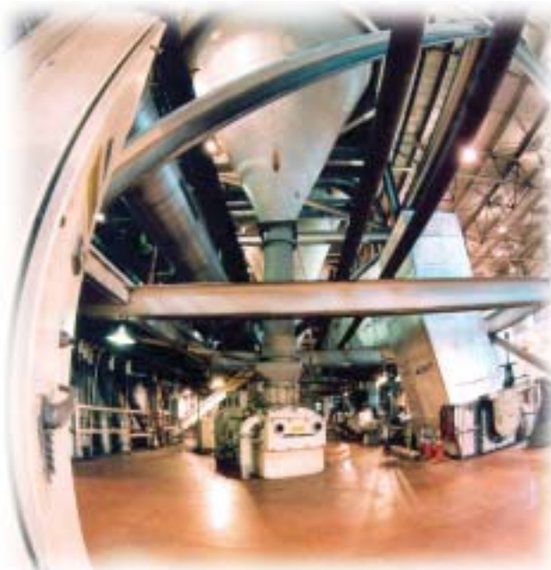
Optimization software from Emerson Process Management provided WE Energies with a cost-effective method of reducing NO x at its Valley Power Plant in Milwaukee. Photo courtesy of Emerson Process Management.
